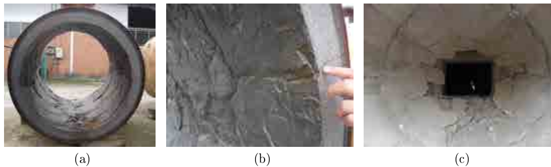
Figure 1.2: Inside the Riser: a) Riser, with concrete covering the steel; b) Crack propagation in the concrete thickness; c) Map crack inside the riser. Source: Personal archive of Professor Eduardo Fairbairn.
